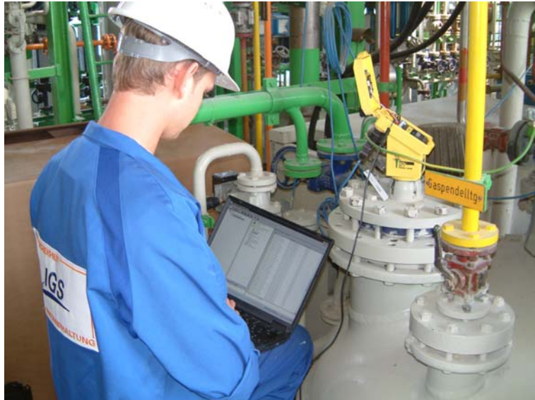
On-site device parameterization by EMR technician from IGS GmbH. In future, he will be able to do this directly from his workstation at the workshop.
